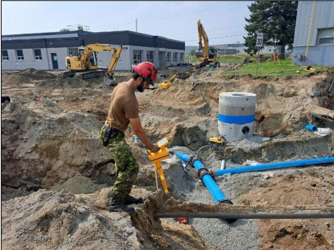
Cpl Mithra Tanskanen performing cable locates after a broken water main in North Bay.
